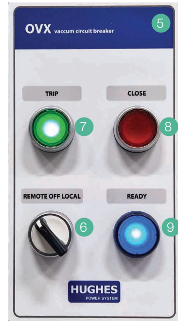
Electrical operation and indicator panel
